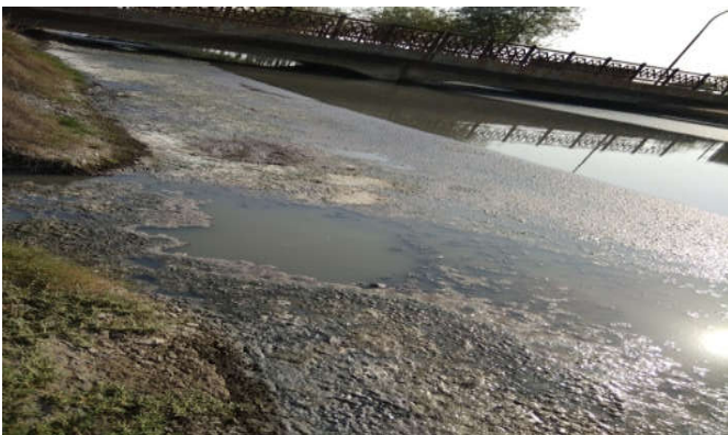
Figure 2. Outlet meshed with solid garbage of CLC.
